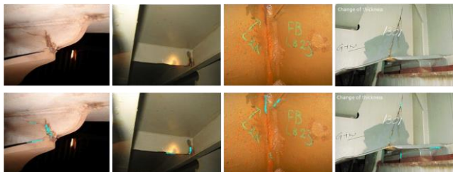
Figure 9: Examples of corrosion-guided crack detection: [top] original images, [bottom] processed images (cracks indicated in light blue).
