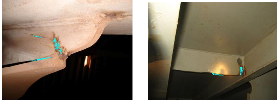
Fig. 12. Cracks detected by GPCD.
