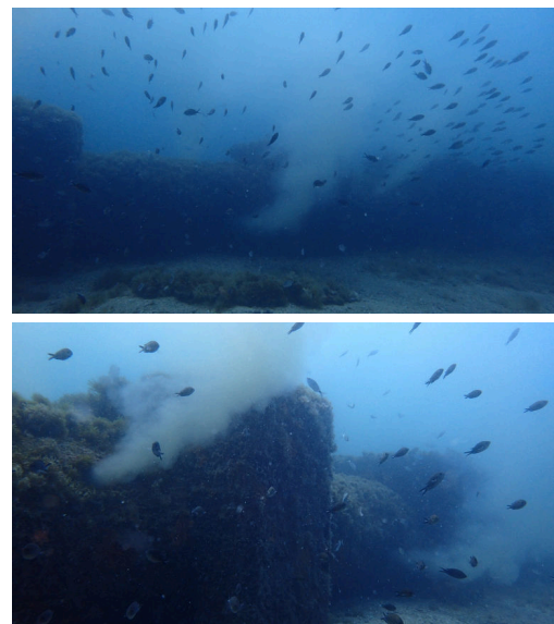
Fig. 3: Two images showing the Palma sewage pipe with two holes in it. Courtesy of Juan Poyatos Oliver et al .
